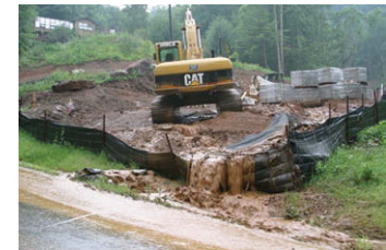
Citizen training programs aim to reduce erosion on construction sites. See page 14.
