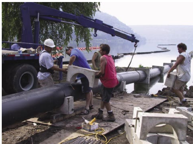
Concrete weights attached to the pipe keep it on the lake bottom.
