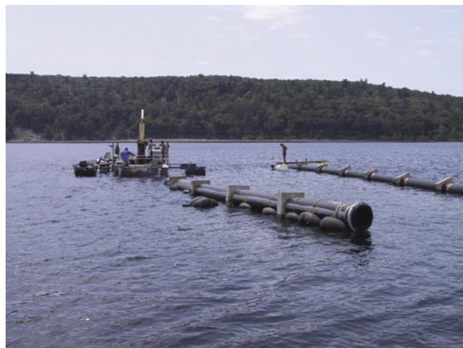
A barge helps position the pipe intake at the deepest part of the lake.
