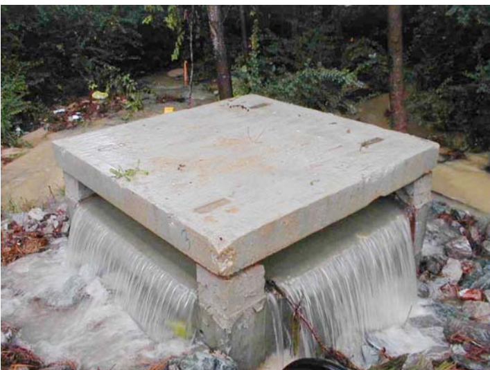
In Aberdeen, NC, a compact weir releases water on all sides, distributing stormwater to bioretention cells.
