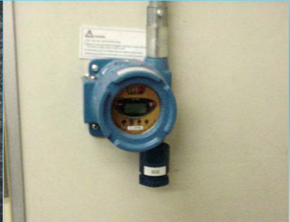
Fixed detectors located in 7 locations in building to detect excess So 2 levels
