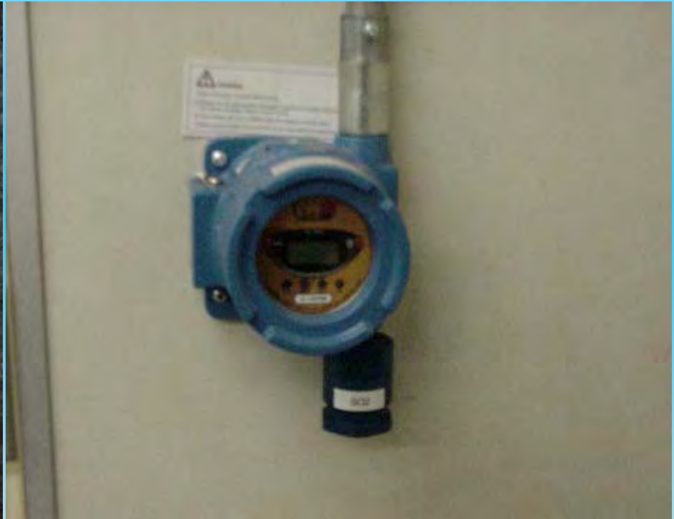
Fixed detectors located in 7 locations in building to detect excess So 2 levels
