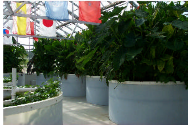
Wastewater from the school passes through aerated reactors that are filled with tropical plants. The plants are also studied during botany lessons.
