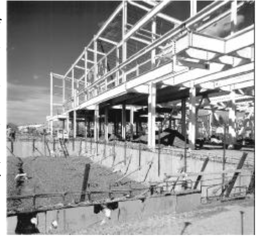
"Photo Copyright © 2003 James S. Vénis. All rights reserved." Construction of the Light Rail Facility is Underway
