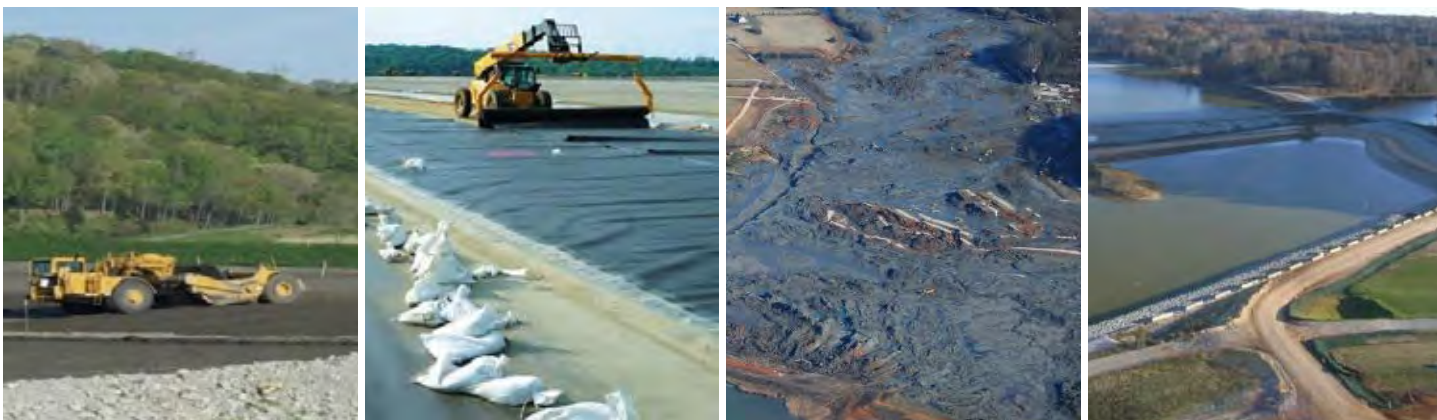
Left to right: Cleanup work, cap installation, and a before and after view of the Middle Embayment area at the TVA Kingston site.
