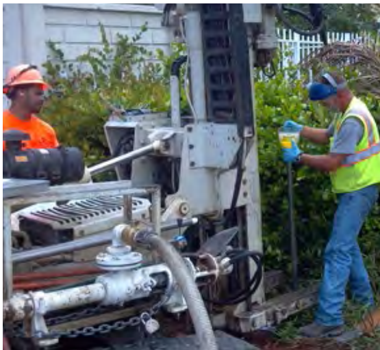
Installation of an injection well for groundwater cleanup at the Flash Cleaners site.
