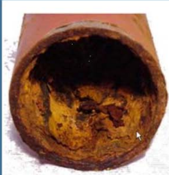
Rusted iron water pipe
