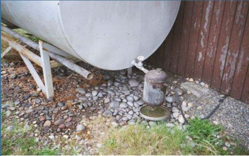
Fuel tank leaking diesel next to wellhead Credit: Rural Community Assistance Corporation
