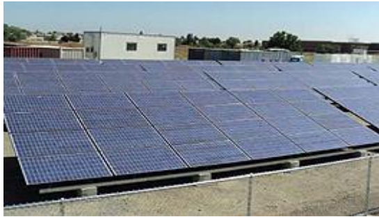
Ground-mounted solar photovoltaic system installed at the Frontier Fertilizer Superfund Site, Davis, California. (EPA photo)
