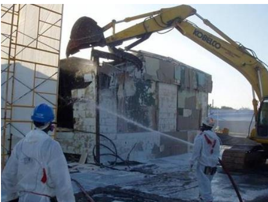
Demolition and wetting of an Alternative Asbestos Control Method building. (EPA photo)
