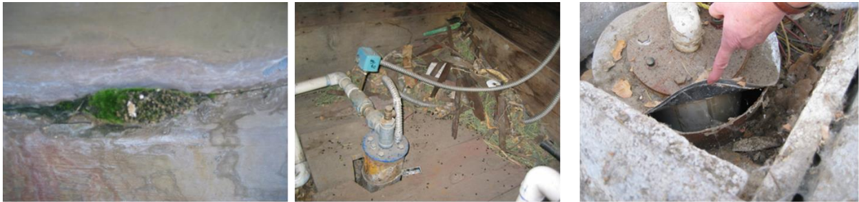
Cracks on a storage tank Rat droppings around the wellhead Seal on wellhead not watertight
