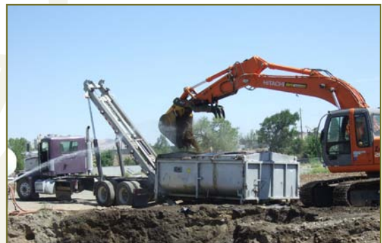
Soil remediation taking place at the future site of Three Nations Plaza in Reno, Nevada.
