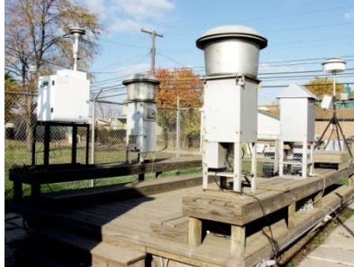
Equipment at a typical regulatory monitoring site.
