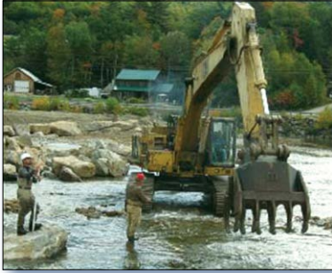
Figure 2. Construction contractors and the project's fluvial geomorphologist used heavy equipment to construct in-stream features.
