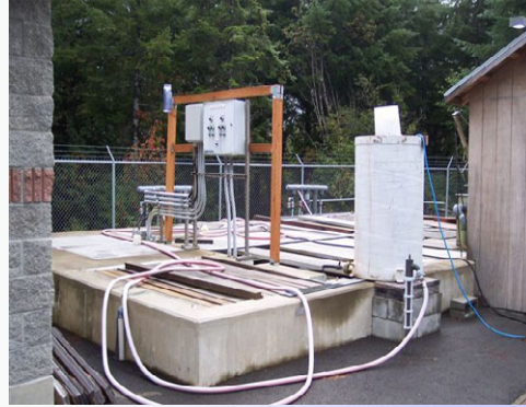
Small wastewater treatment plant
