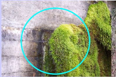
Leaking reservoir wall
