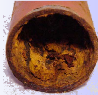
Rusted iron water pipe
