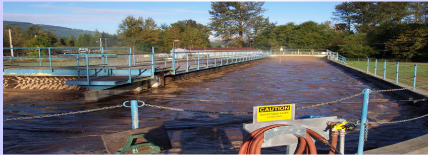
Credit: City of North Bend, Washington WWTP; Sewer Division
