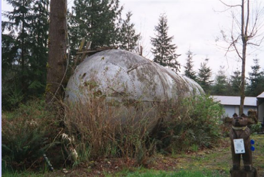
Poorly maintained reservoir
