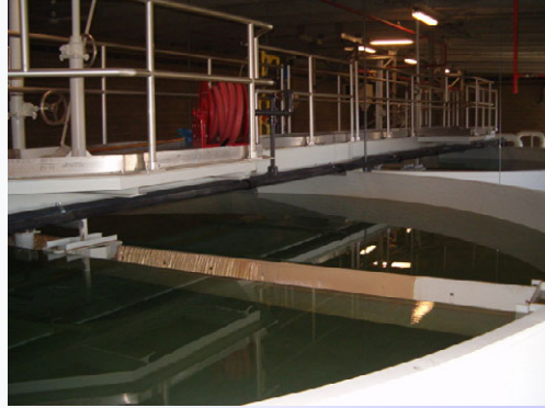
Small drinking water treatment plant Credit: Village of Forsyth, IL
