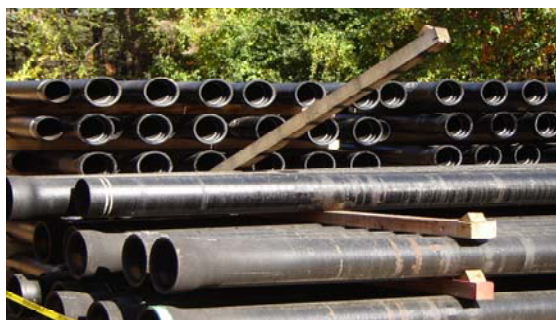
Pipes for water main extension project, Goffstown, New Hampshire. (EPA OIG photo)
