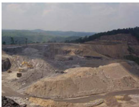
Fill from surface mining operations may be discharged into surface waters or wetlands. (EPA photo)
