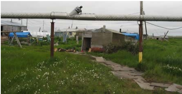
Sewage pipe system in an Alaska village. (EPA photo)
