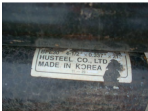
Grouting pipes for the Gilt Edge Mine Superfund site project labeled Made in Korea . (EPA OIG photo)
