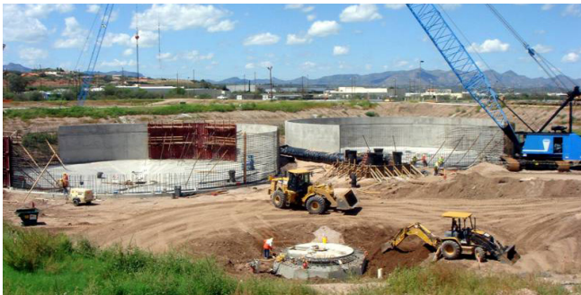
Construction at the Nogales International Wastewater Treatment Plant in Rio Rico, Arizona (EPA photo).
