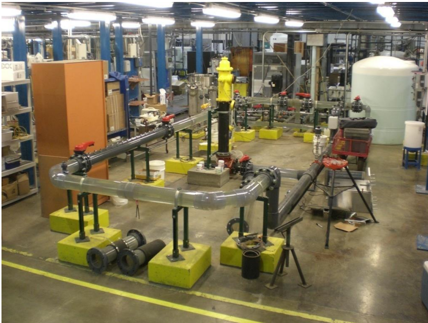
Clear PVC pipe with sampling ports and fire hydrant
