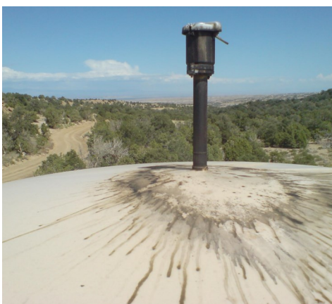
Hydrocarbon staining under a PRV indicating storage vessel over-pressurization.
