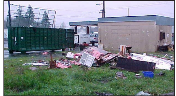
The abandoned gas station site, prior to cleanup.
