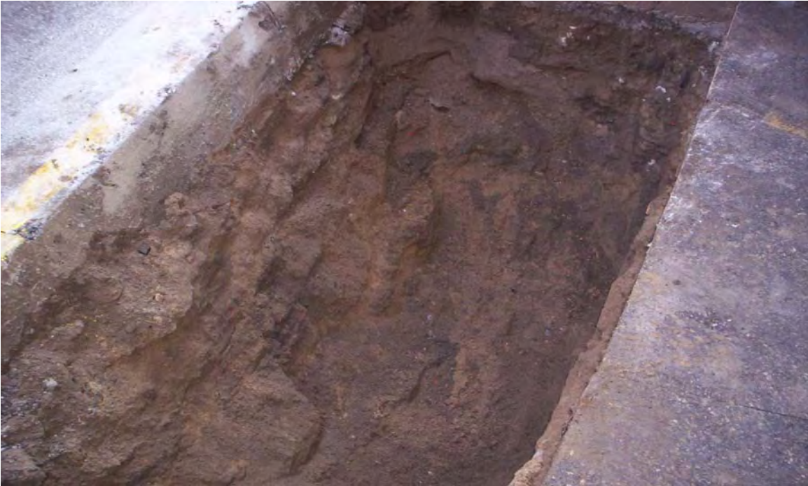
Photo 8: Taken south to north. Shows completion of test pit #2 with no utilities present.
