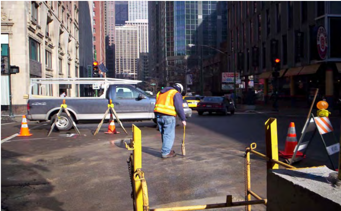
Photo 3: Taken south to north. Shows radiation walkover survey above location of test pit #1 prior to beginning excavation.
