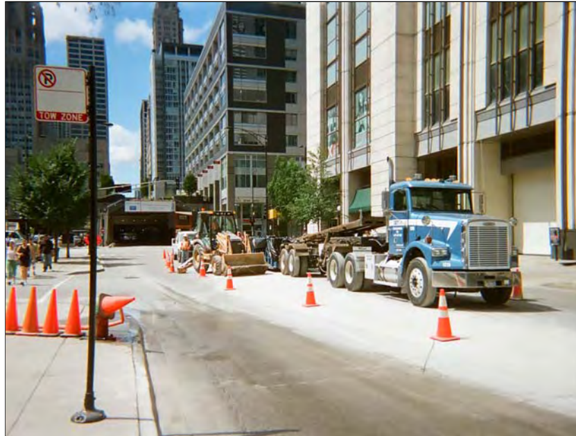
Photo 1: Taken east to west. Shows planned trench run along Illinois Street prior to the beginning of excavation.
