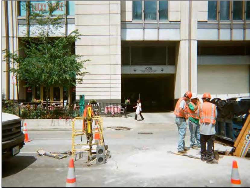
Photo 3: Taken south to north. Manhole starting point for trench on Illinois Street at beginning of excavation.
