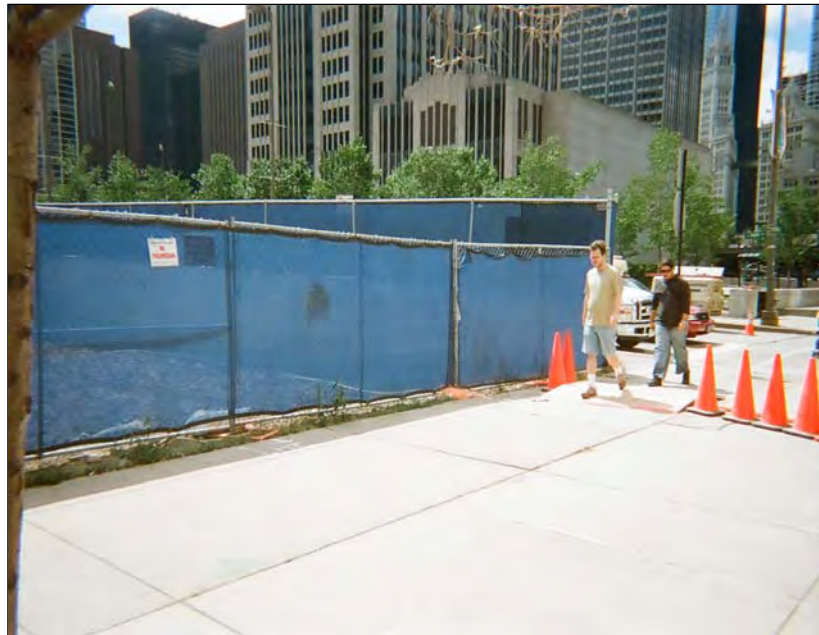
Photo 2: Taken east to west. Conduit tie-in location at property line across sidewalk prior to beginning excavation. Site currently undergoing construction.
