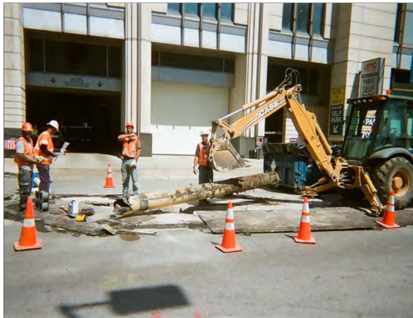
Photo 8: Taken south to north. Removal of out-of-service natural gas main encountered during excavation after cutting into sections.
