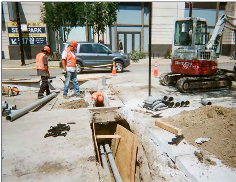
Photo 10: Taken south to north. Installation of conduit pipes in north to south trench section at the completion of excavation and radiation monitoring.
