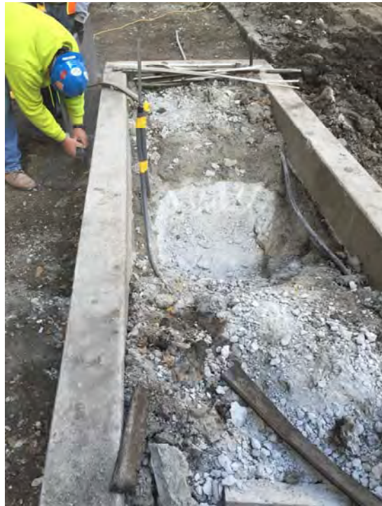
Photo 2 – Tree root-ball excavation for planters located above the concrete slab covering the former slip.
