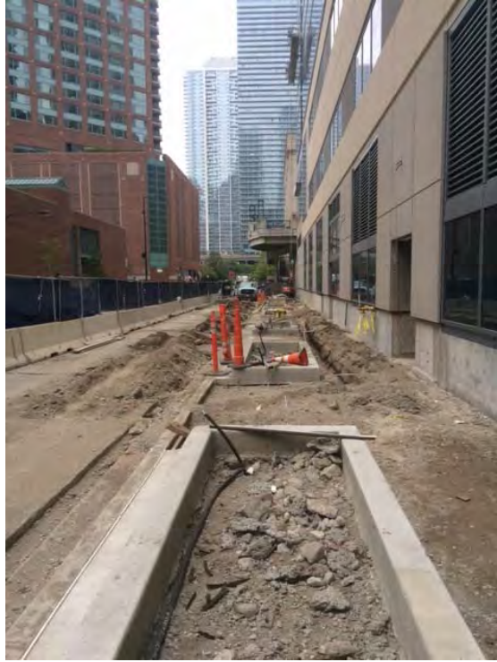
Photo 1 – Looking south along western sidewalk on N. New Street at planters and electrical trench in sidewalk.
