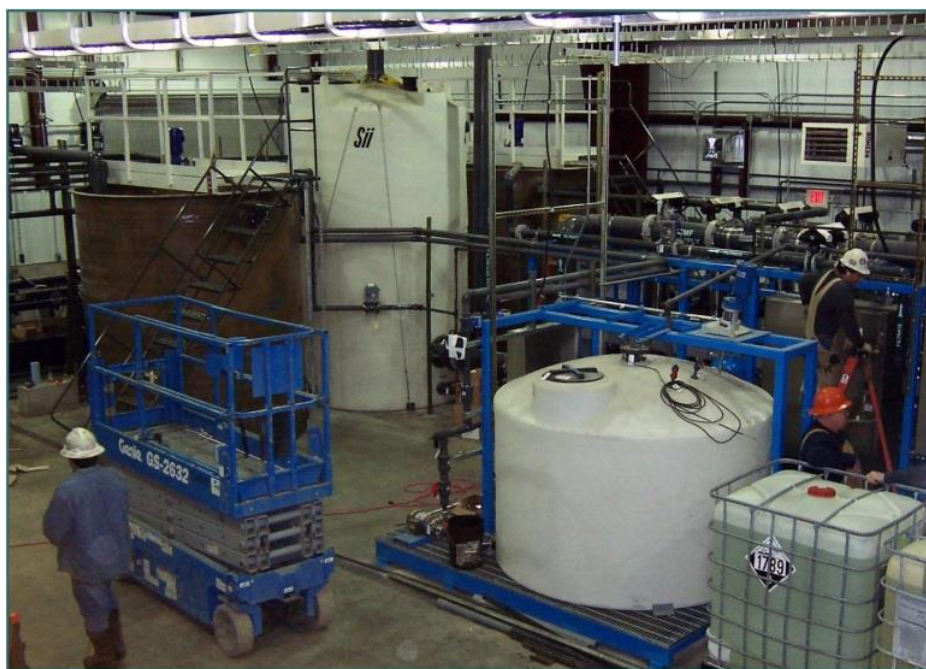
Figure 21: Ceramic Microfiltration System at the Upper Blackfoot Mining Complex, Montana
