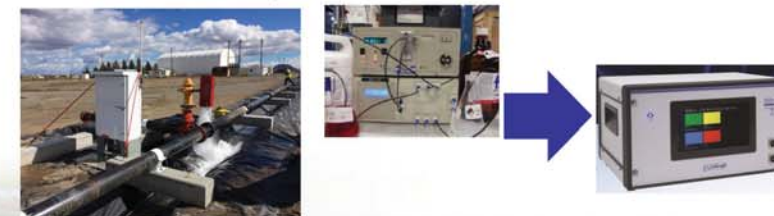
Automated Flushing Hydrants and On-line Monitoring Testing/Development for Rapid Detection
