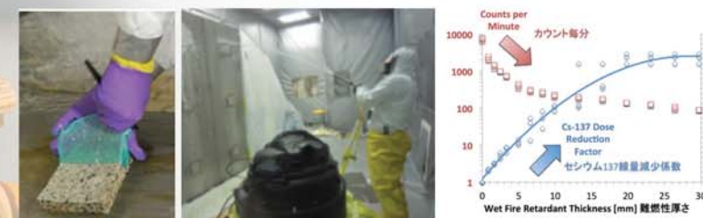
Examples of Mitigation Methods (L → R): Strippable Coatings, Foam Application, and Dose Reduction as a Function of Foam Thickness
