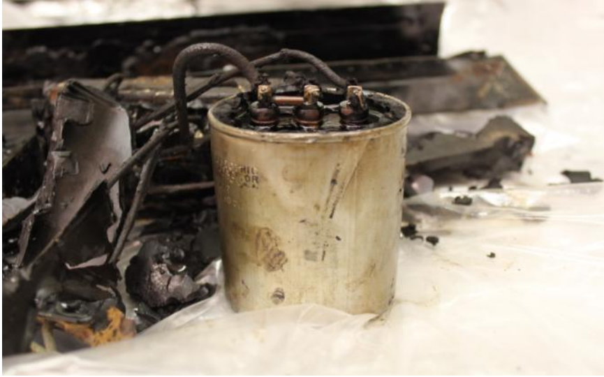
Figure 4.26. Capacitor in ballast BL-02
