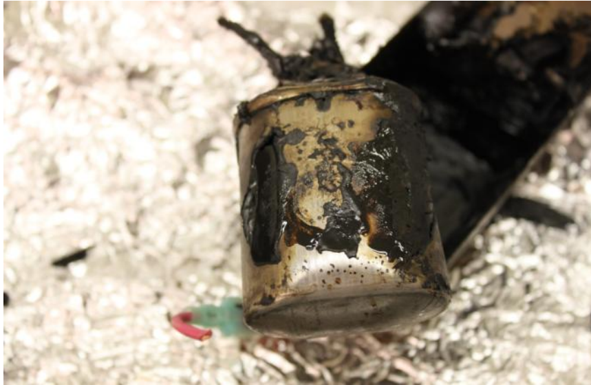
Figure 4.30. The capacitor in the burst ballast (BL-08) (note the expansion on both ends likely due to the instantaneous high pressure)
