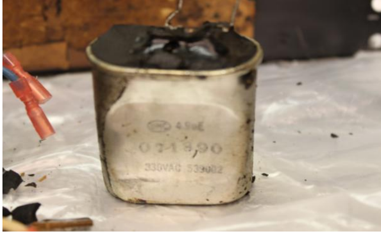
Figure 4.28. Capacitor in ballast BL-02
