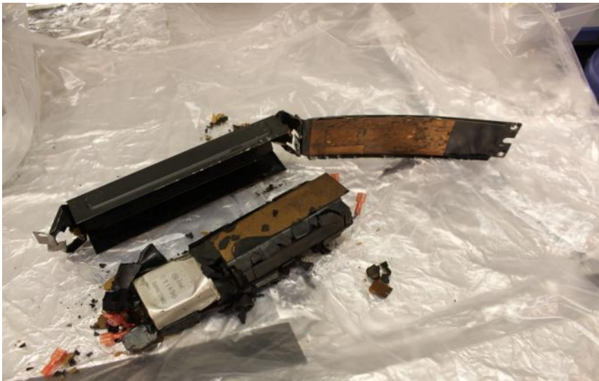
Figure 4.27. Ballast BL-12 after removing the casing (the capacitor is on the left)
