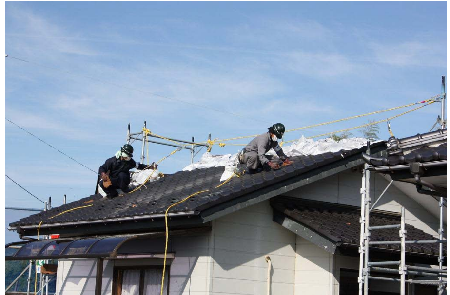
Wiping of roof tiles in Fukushima. Taken from guidelines pertaining to Decontamination and Other Measures
