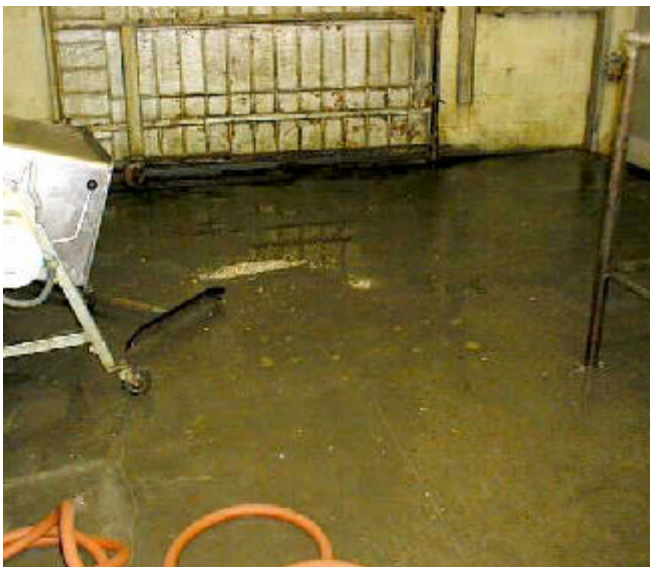
Figure 7. Accumulation of Fat/Meat Trimming Wastes Near a Floor Drain
