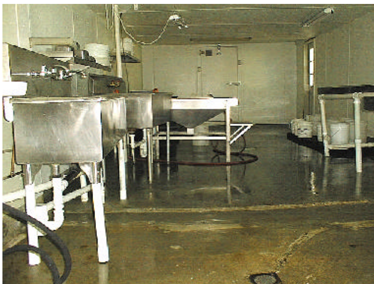
Figure 10. Floor Drains leading to FPWDWs at a Shellfish Processing Facility
