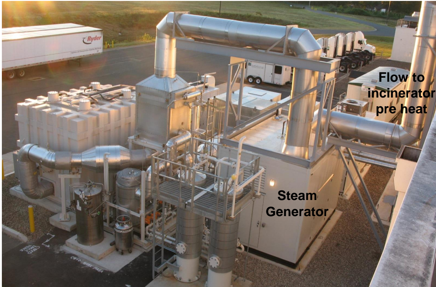
1.2MW Pepperidge Farms, Connecticut Steam generation and incinerator pre-heat for commercial bakery
