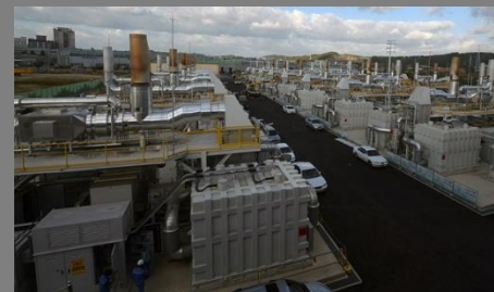
59MW fuel cell park
