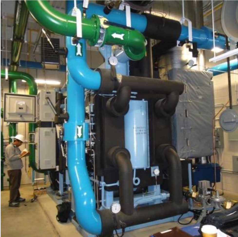
250-ton flue gas fired absorption chiller
