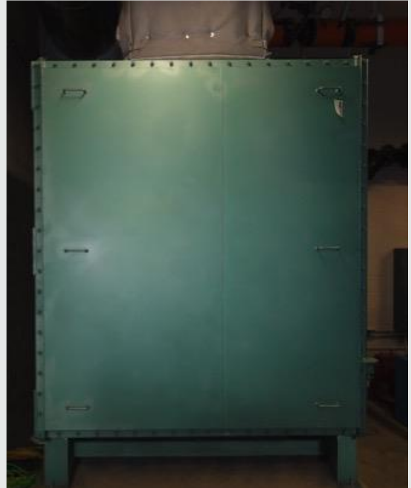
4 MMBTU hot water heat exchanger
