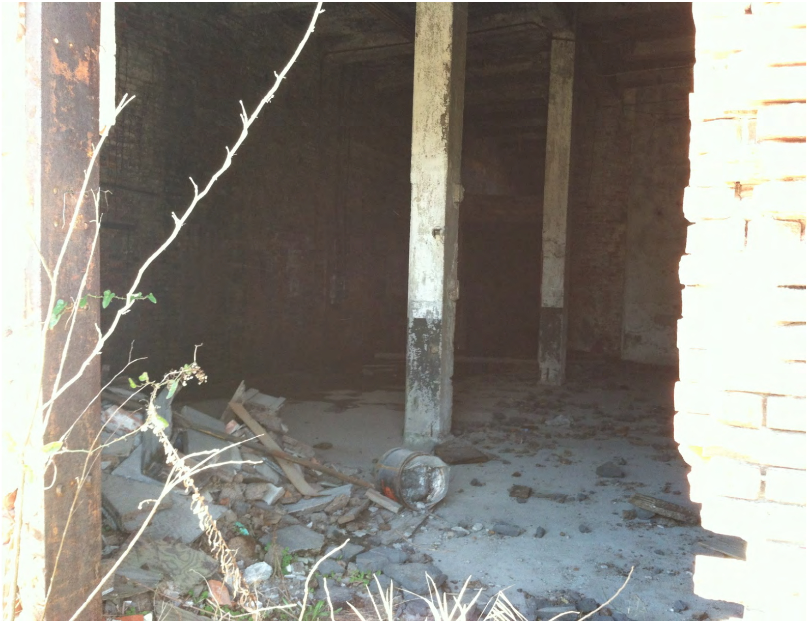
Southern most bay of main building on Peck Iron property. Structural building issues, construction/demolition debris, paint cans and other materials are visible.
