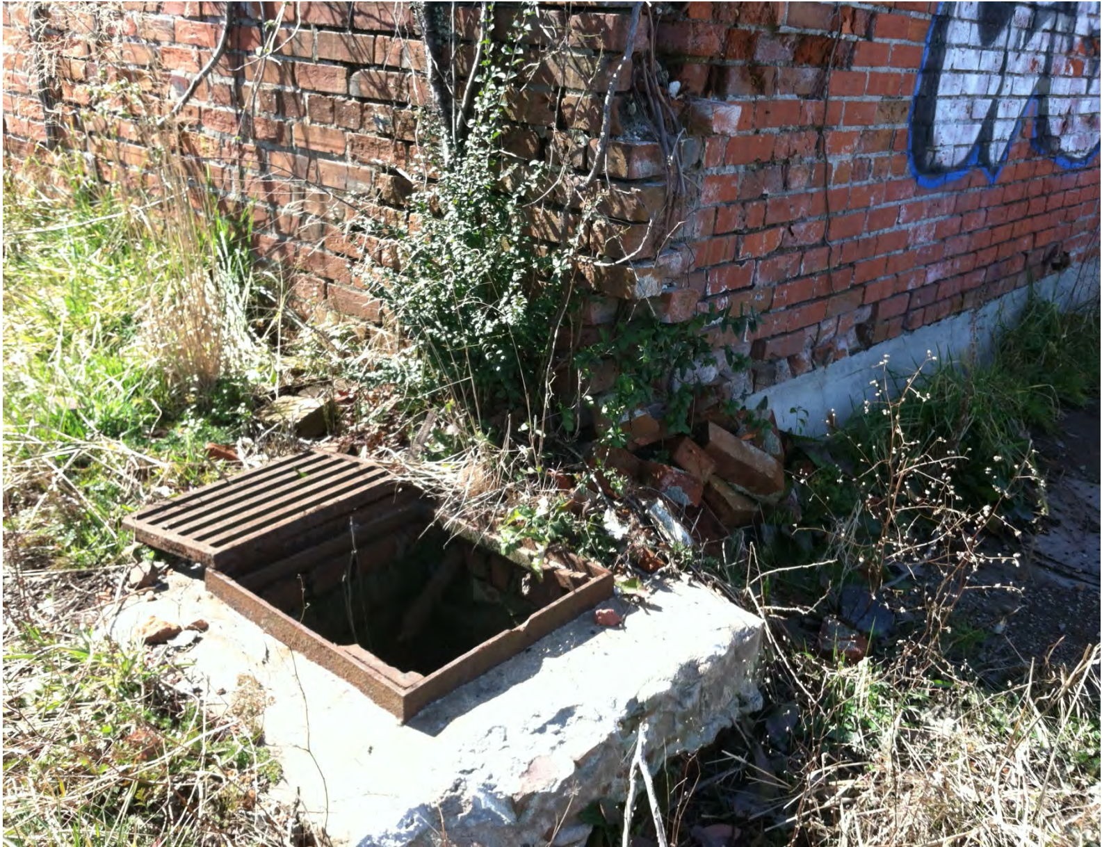
Close up #1 of vat/sump identified at the northeast corner of the main building on the Peck Iron property. Sump was 2-3' deep with ~ 1.5' of standing water and had 2 pipes emanating from the building emptying into this structure.
