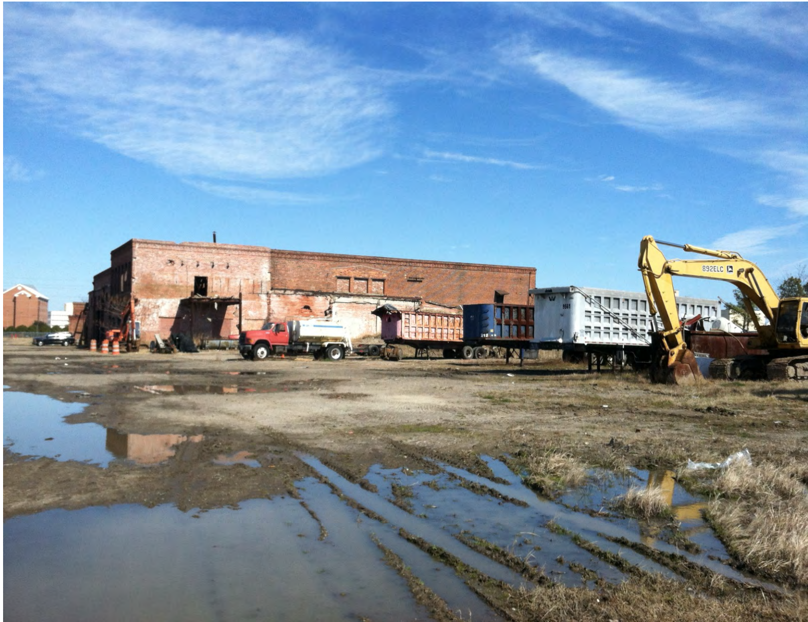
View from south of the main building on Peck Iron property, facing north. Standing water, excavation/trucking equipment, demolition debris piles and other metals debris are located south of the building. On the left side of the photo in the distance to the North you can see the fence bordering the railroad tracks and Elm Avenue property entrance as well as buildings on the north side of Elm Avenue.
