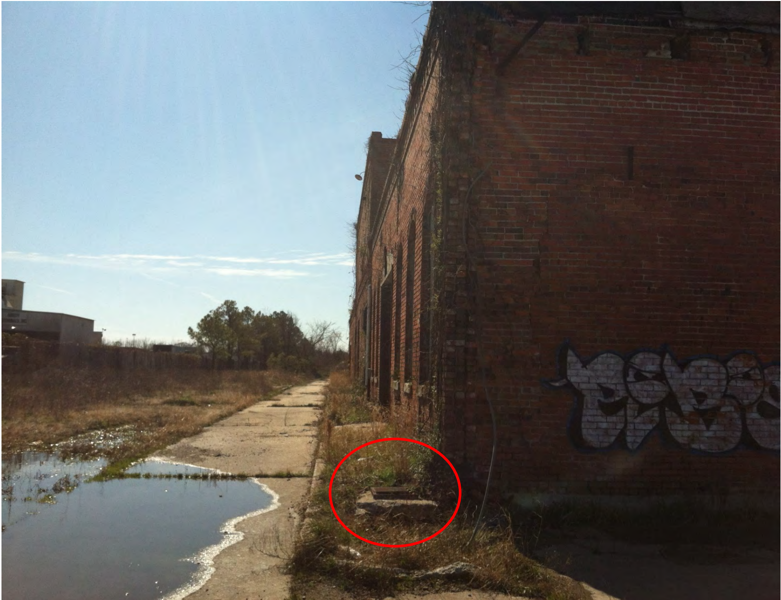
Main structure at Peck Iron property. Northeast corner of building facing South. Vat or sump containing liquid identified at the northeast corner of building.
