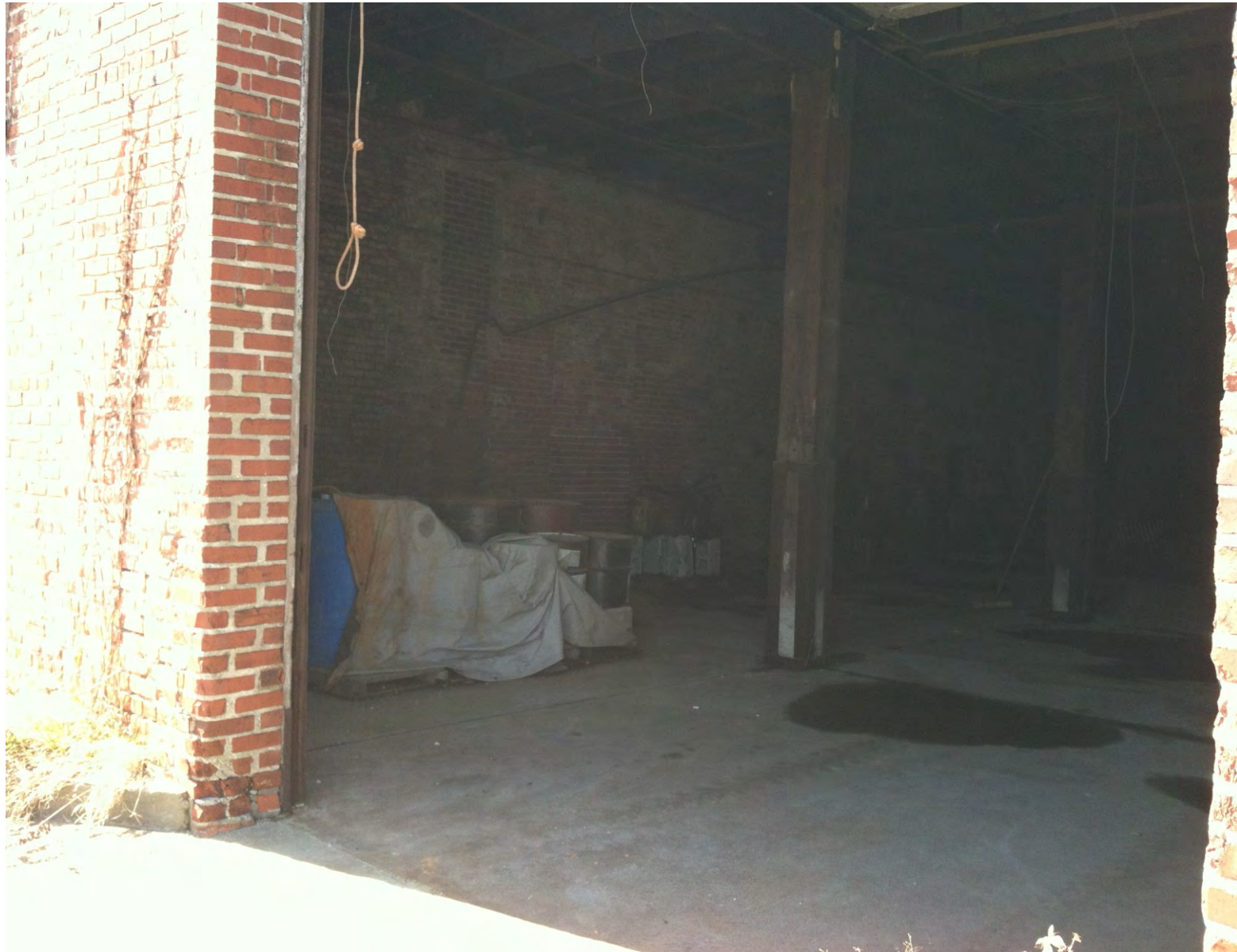
Middle bay of main building on Peck Iron property. Notice drum storage area and staining of concrete areas.
