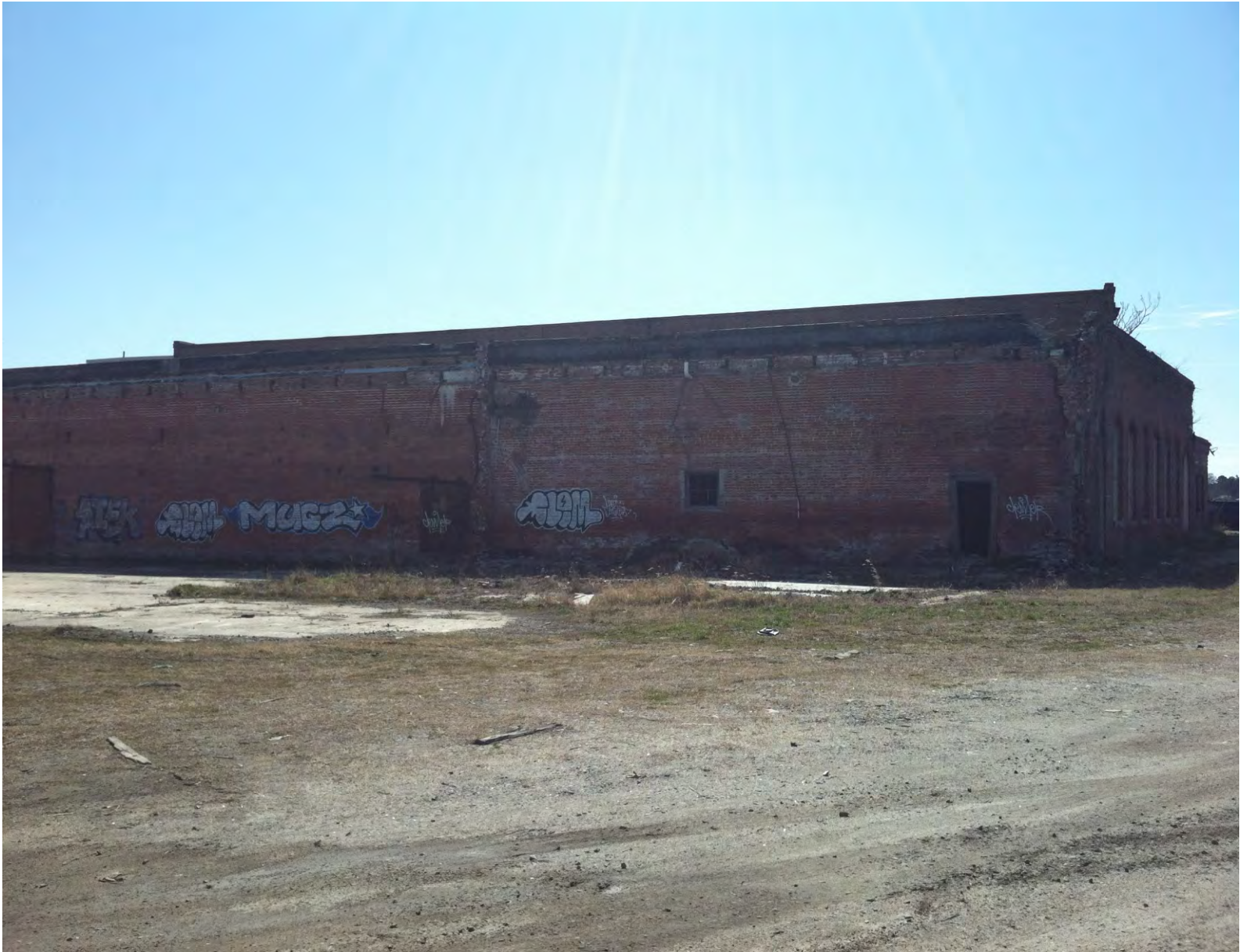
View of the main (largest) structure on the Peck Iron property. Looking south/southeast near entry driveway and access gate. Building is decaying and contains a series of bays used for various storage and auto restoration activities
