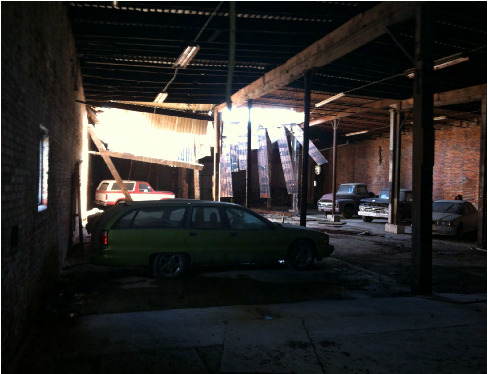
Car storage in the northern most bay of the main (largest) structure on the Peck Iron property. Looking east/southeast, notice roof collapse and other structural issues.
