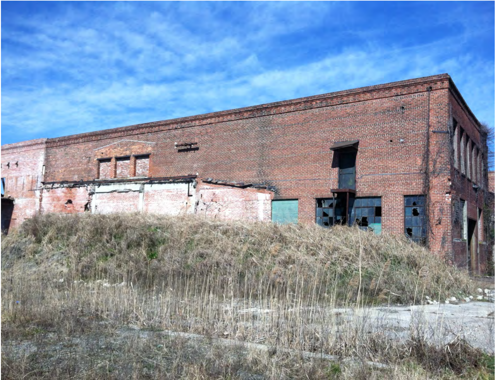
South side of main building on Peck Iron property, facing north/northwest. Demolition debris, excavation equipment and other metals debris are located south of the building.
