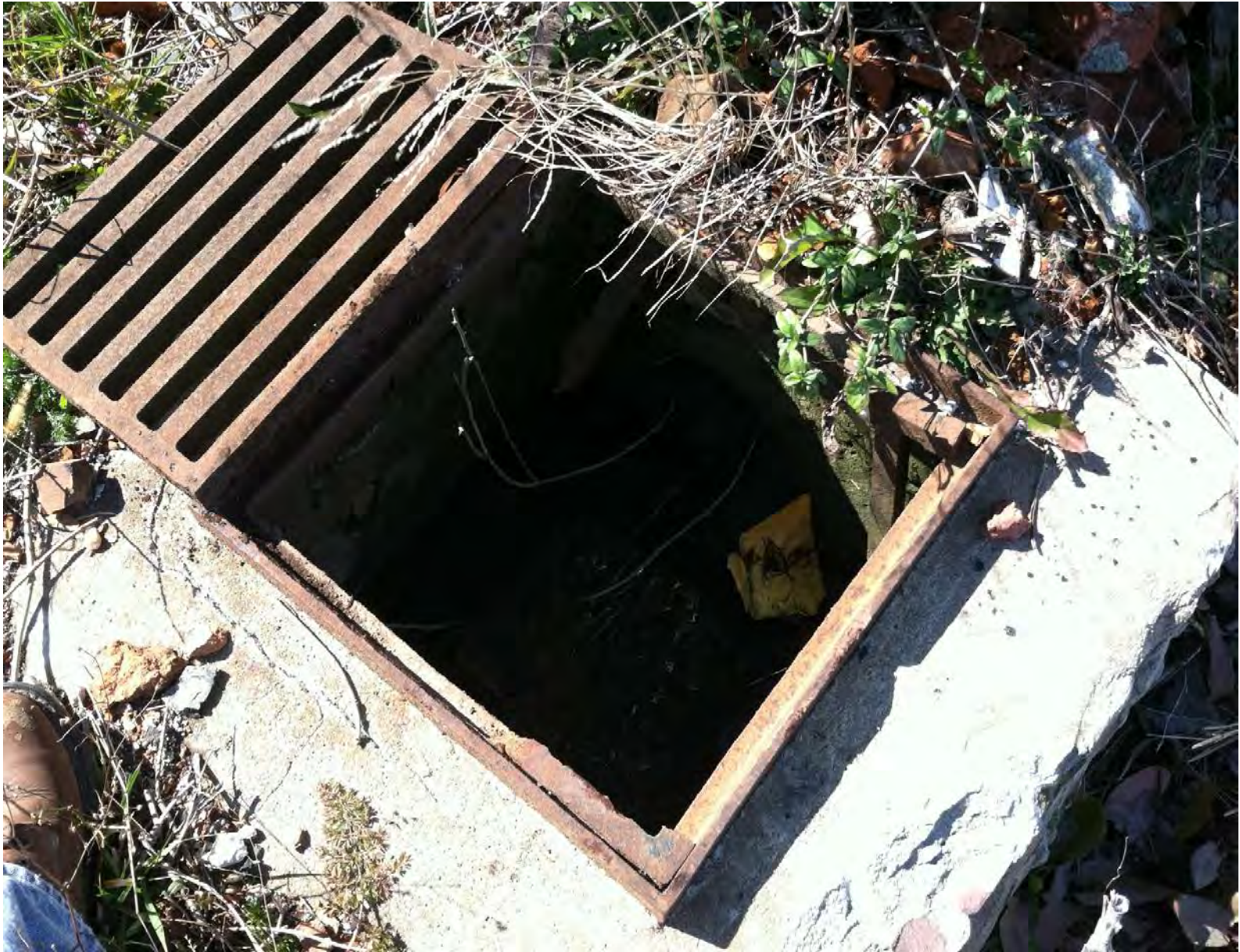
Close up #2 of vat/sump identified at the northeast corner of the main building on the Peck Iron property. Sump was 2-3' deep with ~ 1.5' of standing water and had 2 pipes emanating from the building emptying into this structure.
