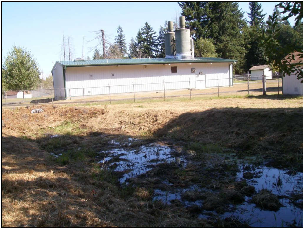
PHOTO 8: City of Tumwater Palermo Well Field – Dual air stripping towers within and above pump house and water treatment building, looking east; note seep drainage in foreground.
