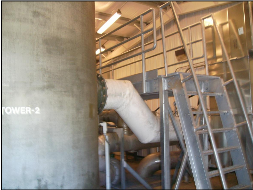
PHOTO 13: City of Tumwater Palermo Well Field – Air Stripping Tower #2.
