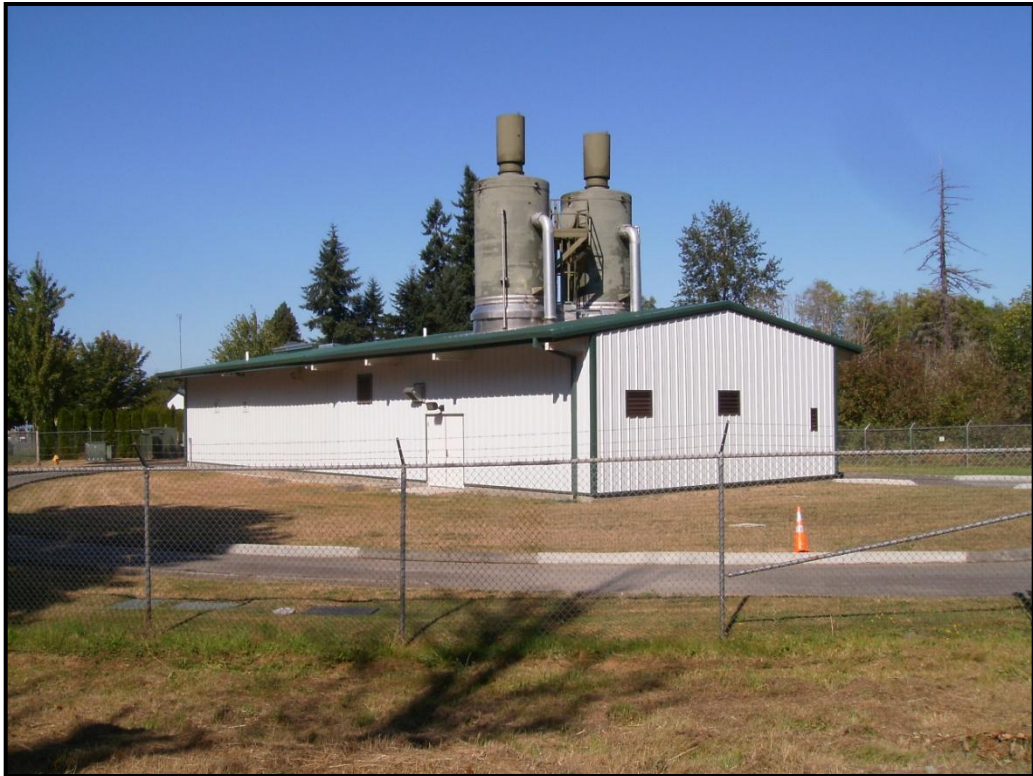
PHOTO 5: City of Tumwater Palermo Well Field – Dual air stripping towers within and above pump house and water treatment building, looking northeast.
