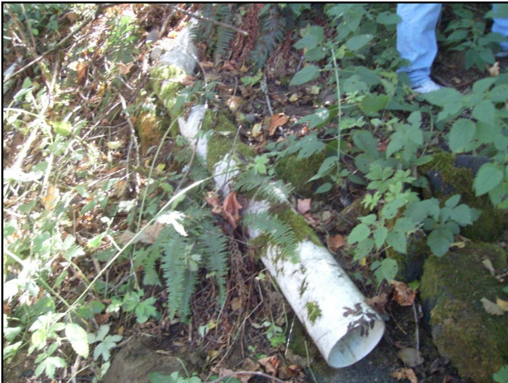
PHOTO 30: 8-inch diameter PVC pipe day-lighting along bluff west of residential neighborhood; location estimated to be 60 feet west of the northwest corner of House #4.
