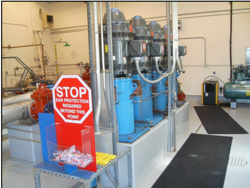
PHOTO 12: City of Tumwater Palermo Well Field – Interior of Pump House.
