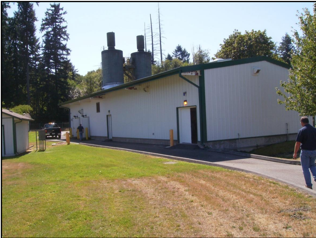
PHOTO 6: City of Tumwater Palermo Well Field – Dual air stripping towers within and above pump house and water treatment building, looking southwest.
