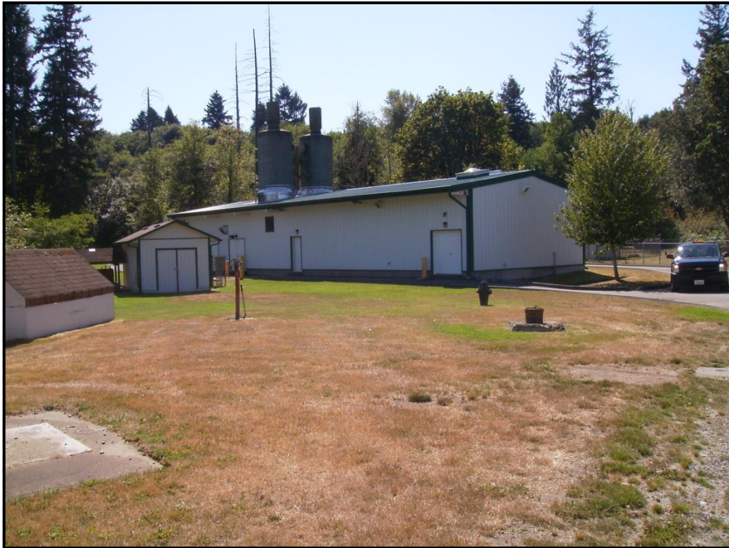
PHOTO 7: City of Tumwater Palermo Well Field – Dual air stripping towers within and above pump house and water treatment building, looking southwest.
