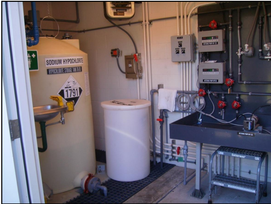
PHOTO 14: City of Tumwater Palermo Well Field – Chemical treatment container (sodium hypochlorite) - typically not used - air strippers used instead to adjust pH.
