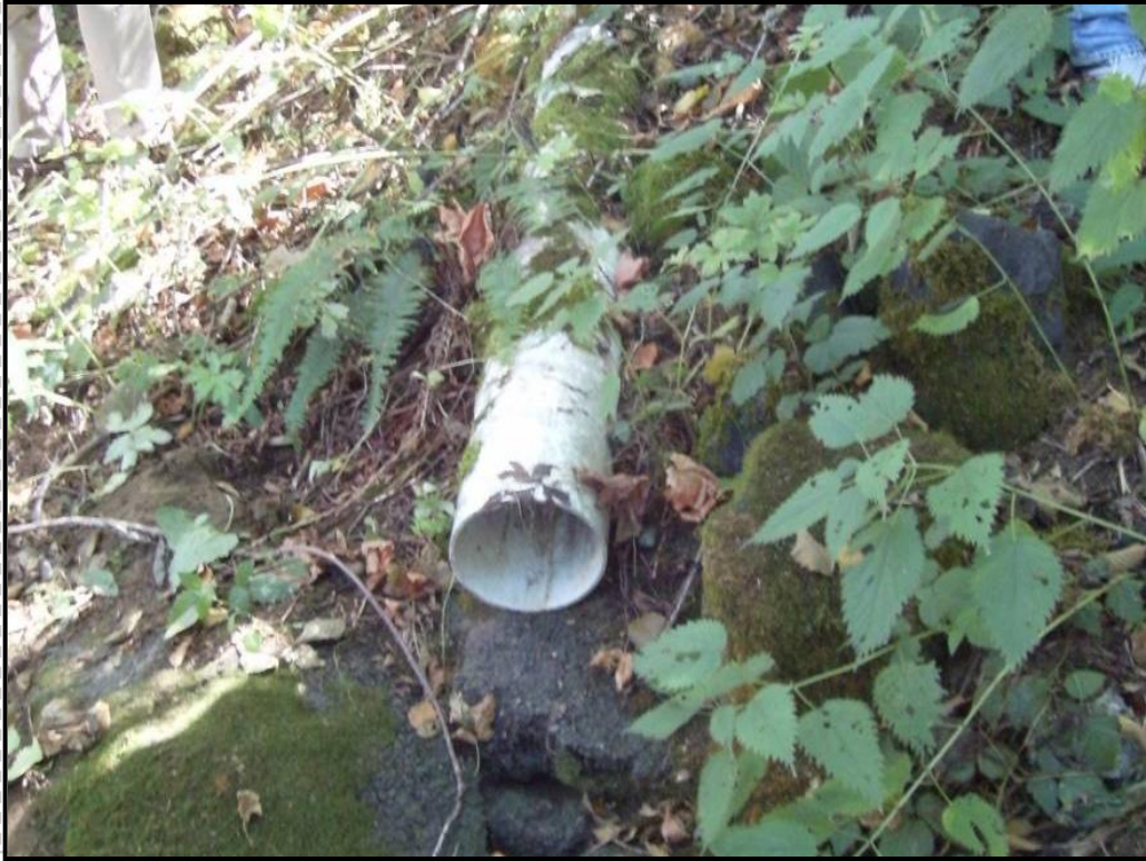
PHOTO 31: Another view of 8-inch diameter drainage pipe along bluff.
