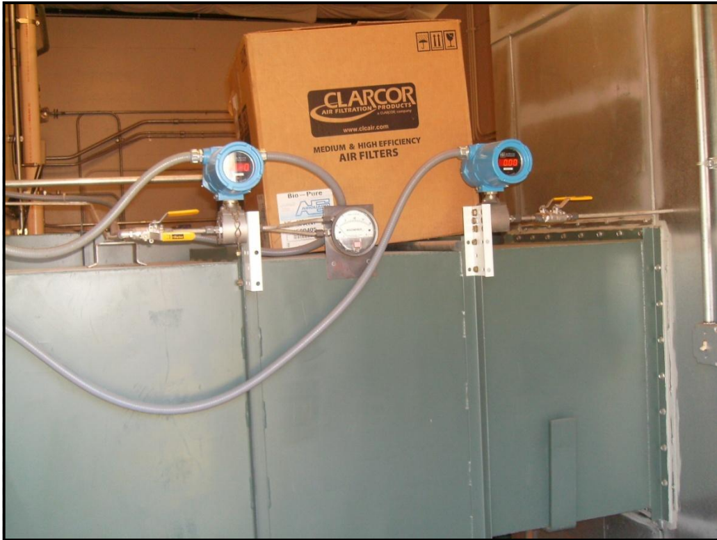
PHOTO 15: City of Tumwater Palermo Well Field – Air ducting for Blower No. 2 for Air Stripping Tower No. 2
