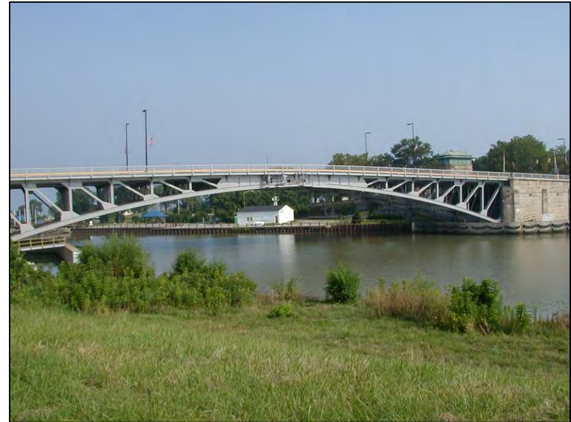
The Bascule (Erie Street) Bridge lies near the mouth of the Black River in Section 1.
