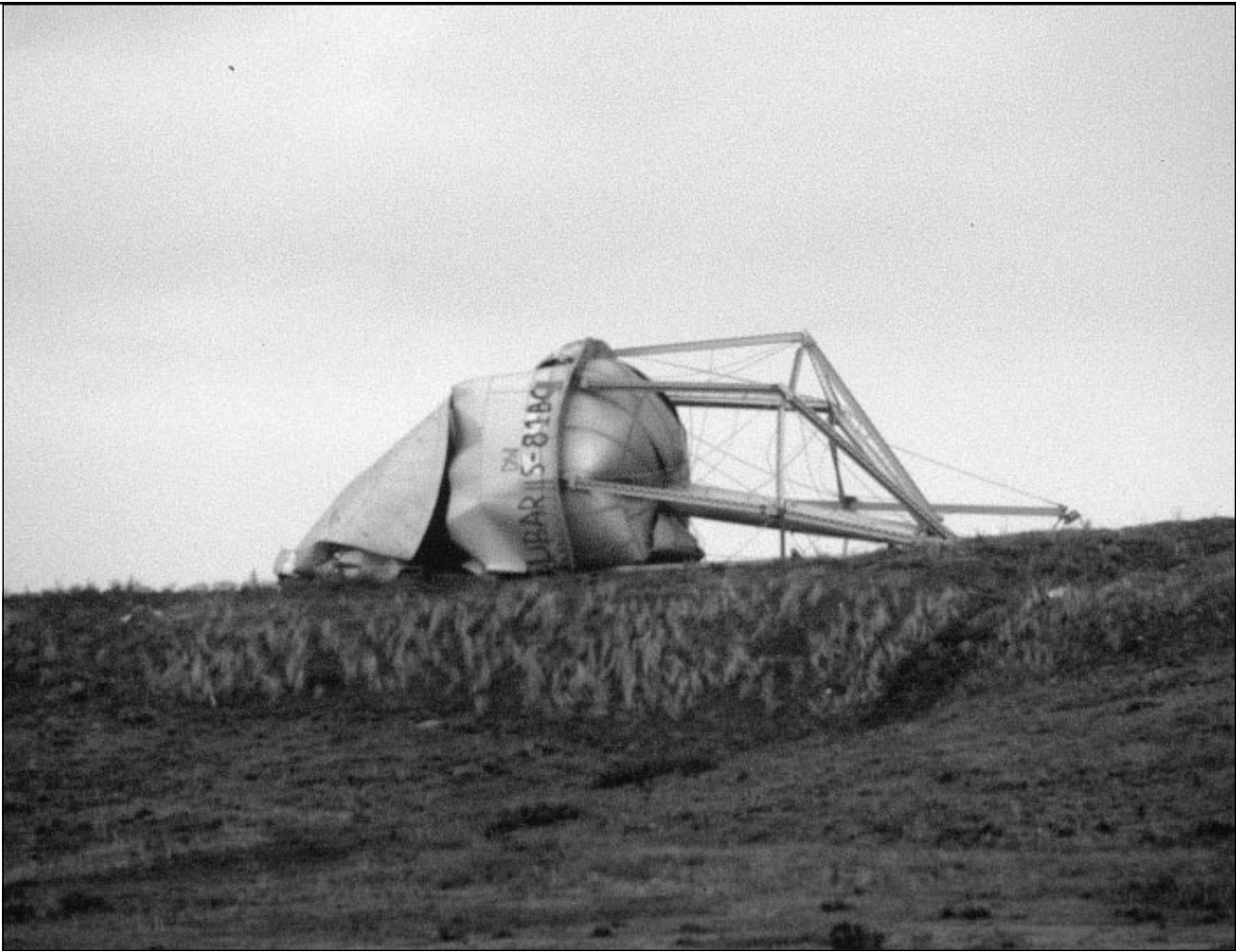
This partially demolished million gallon elevated storage tank had exceeded its useful service life. Needs Survey respondents reported that elevated tanks of this size would cost an average of $1 million.
