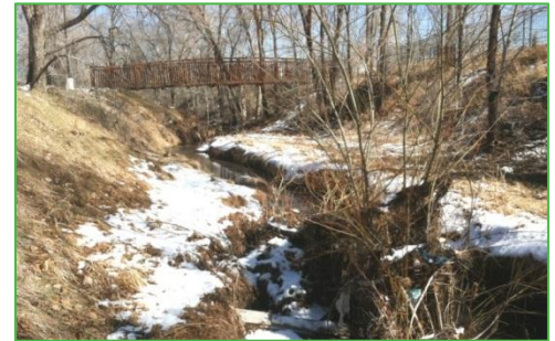
Figure 11: Removal of in-channel debris, reducing erosion potential, flattening channel bank slopes and vegetation maintenance are key project elements in the Dry Gulch channel restoration design.
