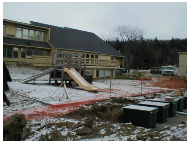
The Warren Elementary School, with a replacement system using alternative technology under construction in the foreground.
