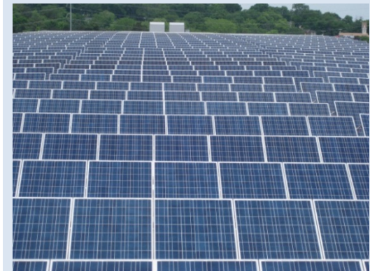
Binkley Solar Farm, Hermitage, TN. Photo courtesy MSCOT Services, LLC.
