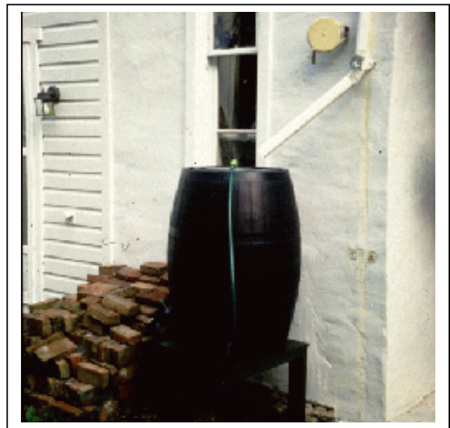
Figure 5.18: A rain barrel that collects runoff from a roof gutter downspout.
