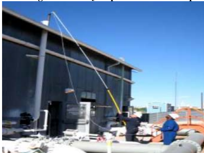
Figure 1: Vent stack leak screening with an electronic gas leak detector, TVA/OVA or infrared gas detector. [See pdf attachment for photo]
