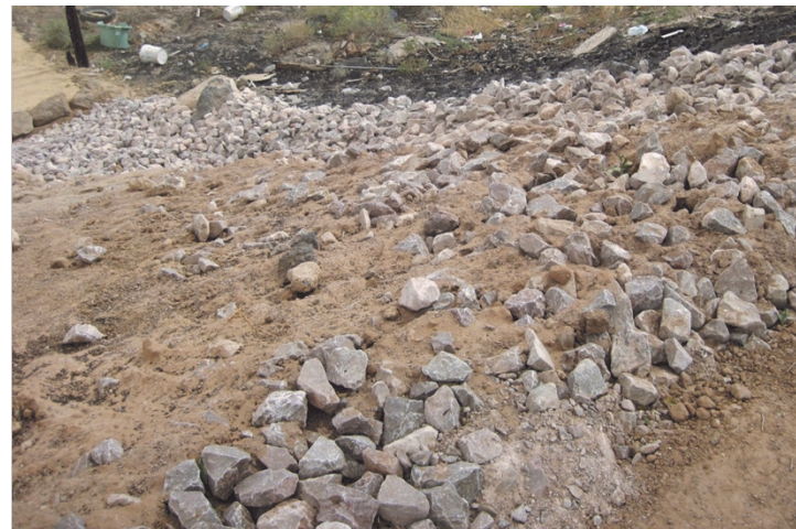
Soil excavation, backfill with clean soil, and rock placement for armoring at residence.
