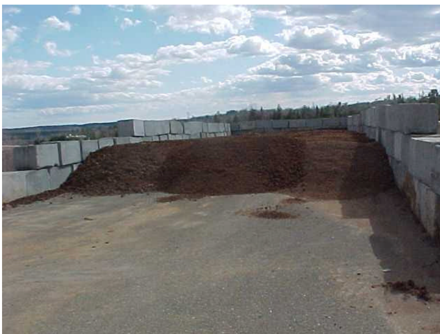
Figure 5-4. Concrete storage bunker with block push walls (Courtesy Mark King, Maine Dept. of Environmental Protection).
