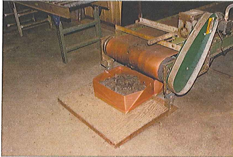
Tritonal Flaking Belt – Building 1619
