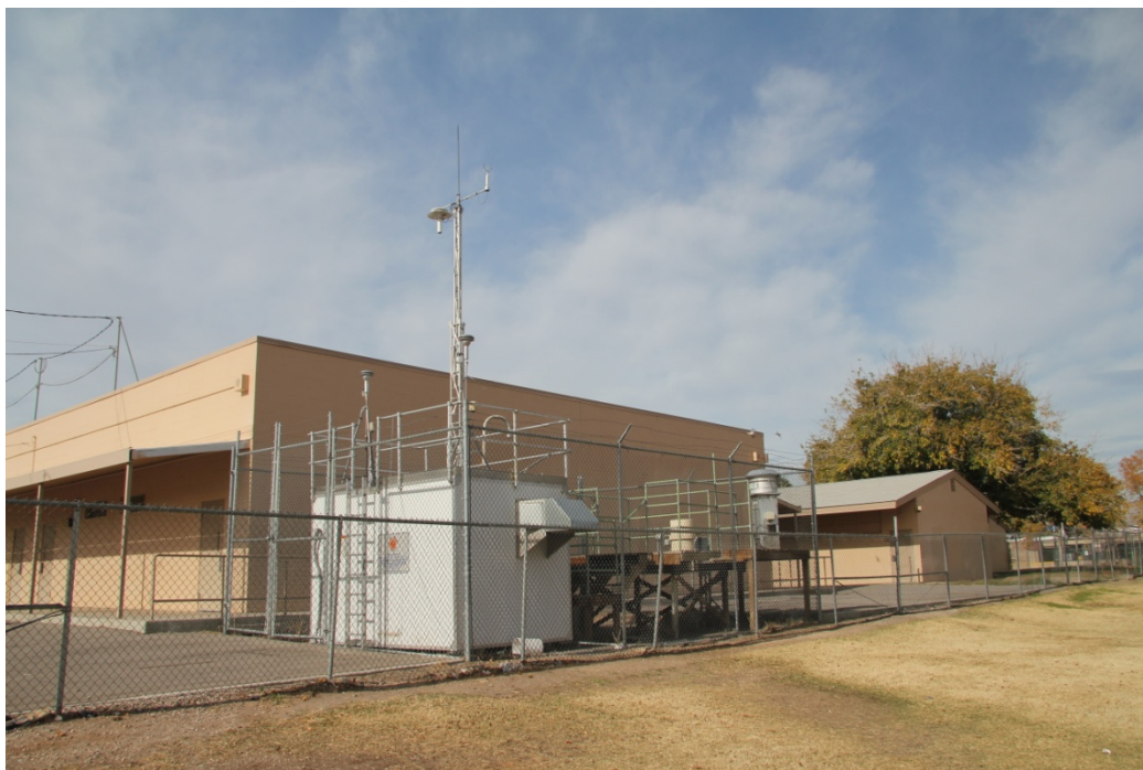
Figure 123. J. D. Smith monitoring station, street view.
