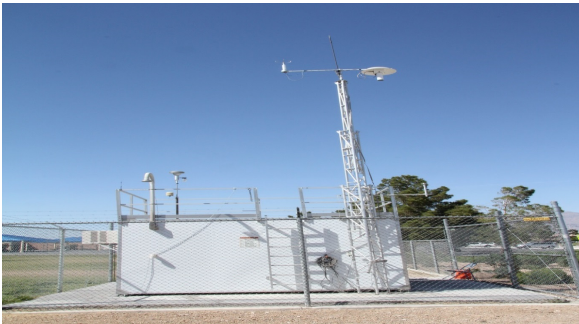
Figure 133. Joe Neal monitoring station, street view.
