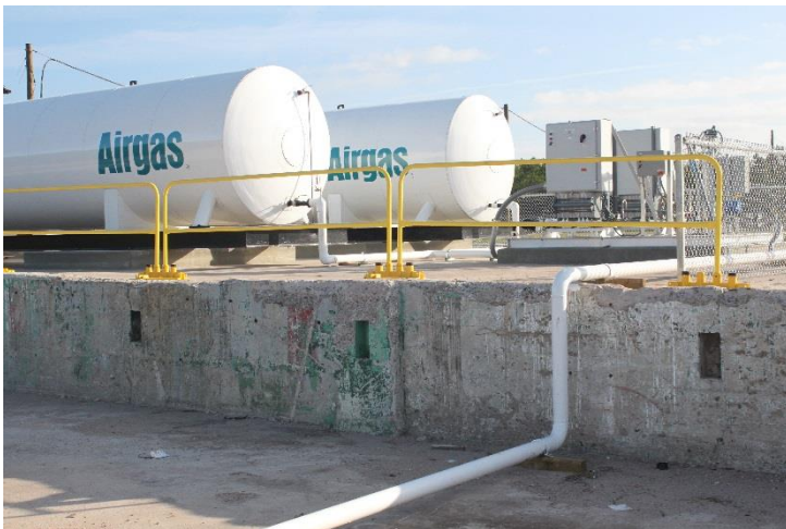
Top left: Typical sparge well. Top right: 105-kw process vaporizers. Middle left: Distribution panel with hose connections. Middle Right: Portable CO 2 sparging system. Bottom left: 50-ton CO 2 storage tanks.
