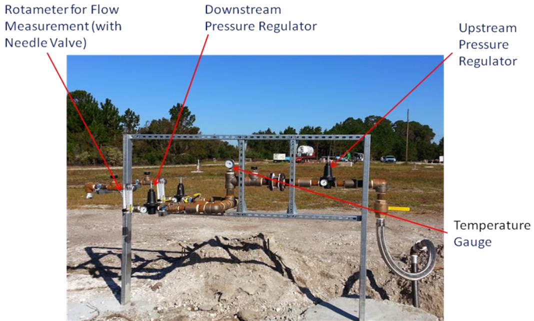
Above: Photo showing a typical distribution panel. Below: Photo showing typical sparge wellhead installation.
