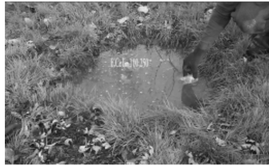
Ponded effluent from a failed septic field
