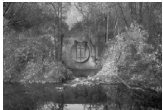
Combined Sewer Overflow
