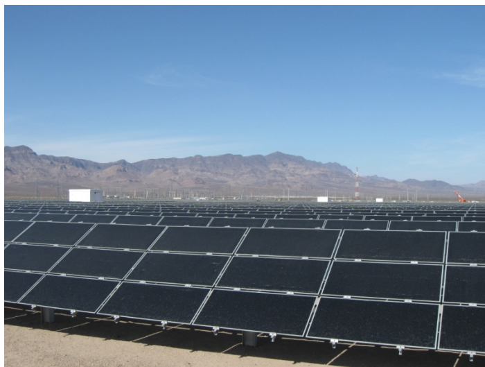
10 MW El Dorado, NV Constructed for Sempra Generation
