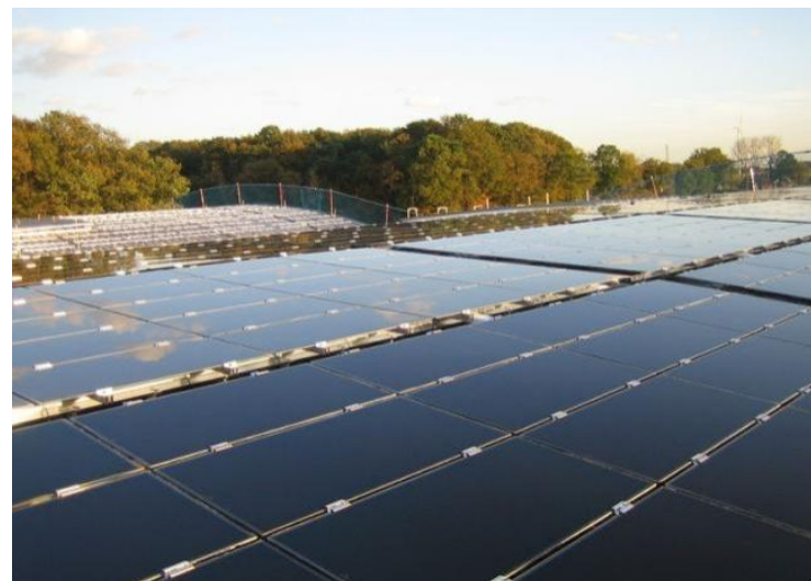
1.4 MW Gescher, Germany Project Developer: Colaxon
