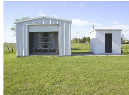
Public water system well and granular activated carbon treatment system
