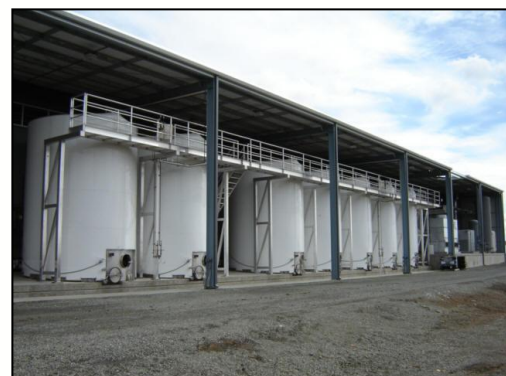
Above-Ground Petroleum Storage Tanks
